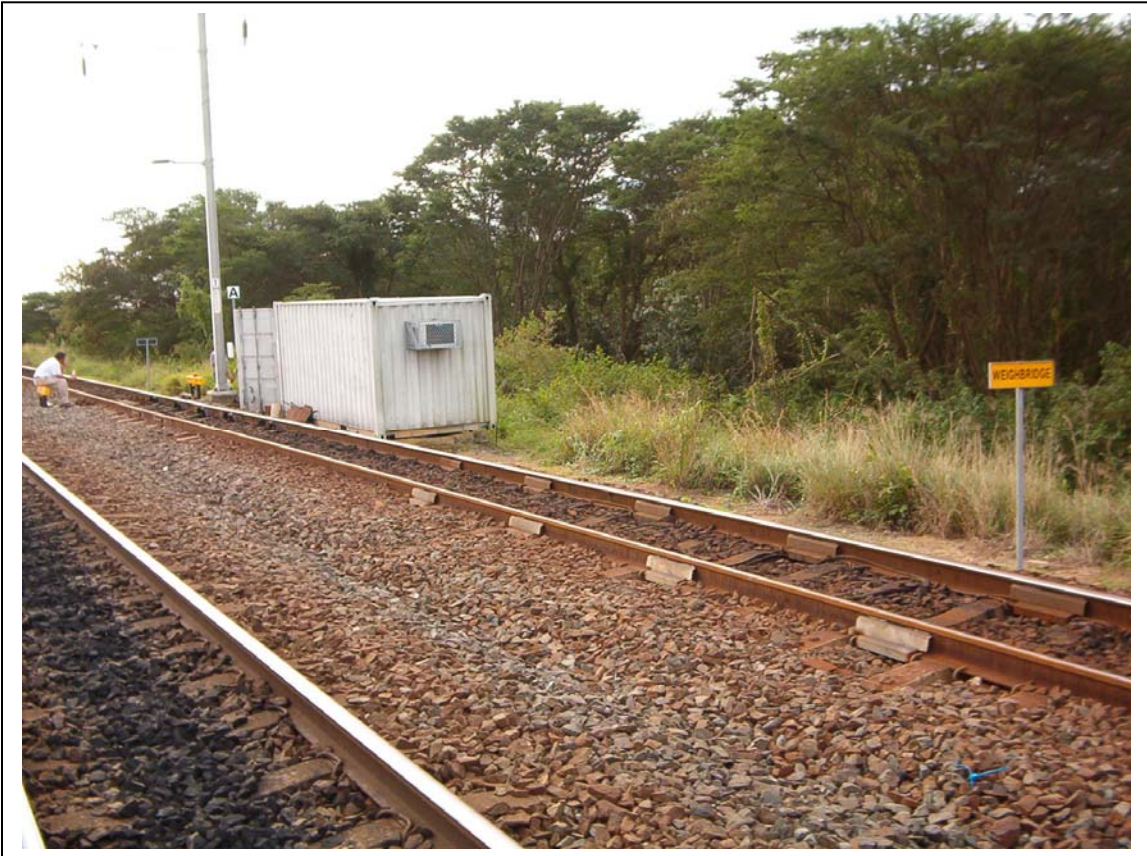
MASSIZE-08 INSTALLION SHOWING SENSORS AND TRACKSIDE ENCLOSURE
